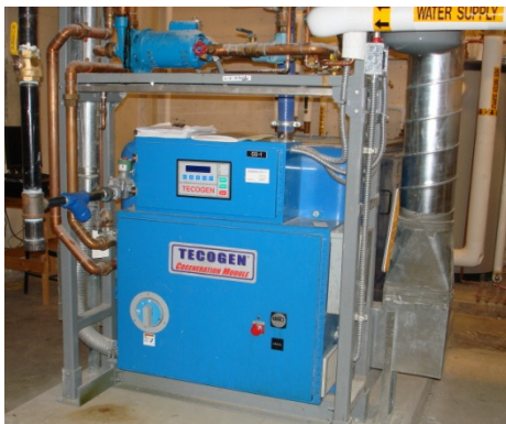
WSU CoGen System
