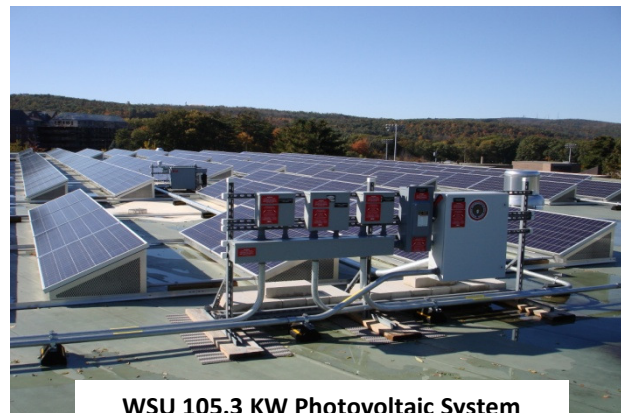
WSU 105.3 KW Photovoltaic System
